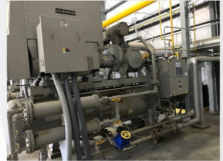
Inlet Gas Compression
