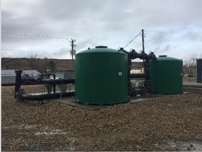
Hydrogen Sulfide Removal
